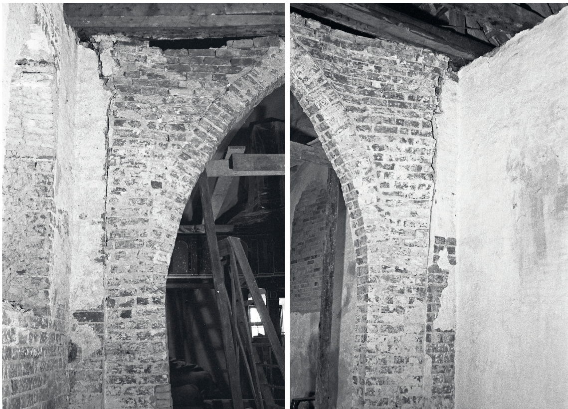
Fig. 66-67. Vanger til \dagger murblandinger i skibets vestmur set mod vest (s. 3922). 66. Sydsiden. 67. Nordsiden. Foto Ebbe Lehn Petersen 1962. I NM. – Side members for \dagger wall recesses in the nave's western wall looking west. 66. South side. 67. North side.
