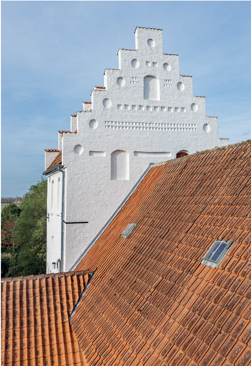
Fig. 18. Tårnets østre taggavl set fra øst (s. 3861). Foto Arnold Mikkelsen 2022. – Eastern roof gable of the tower seen from the east.
