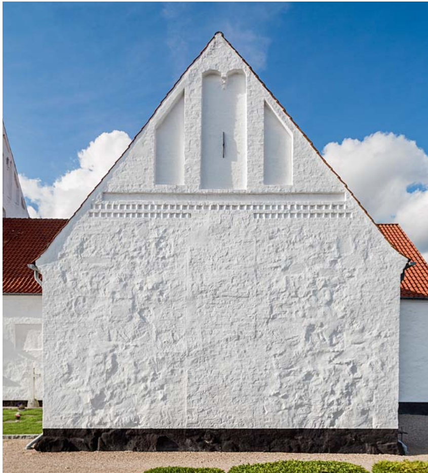
Fig. 17. Søndre korsarm set fra syd (s. 1843). Foto Arnold Mikkelsen 2017. – South transept seen from the south.
