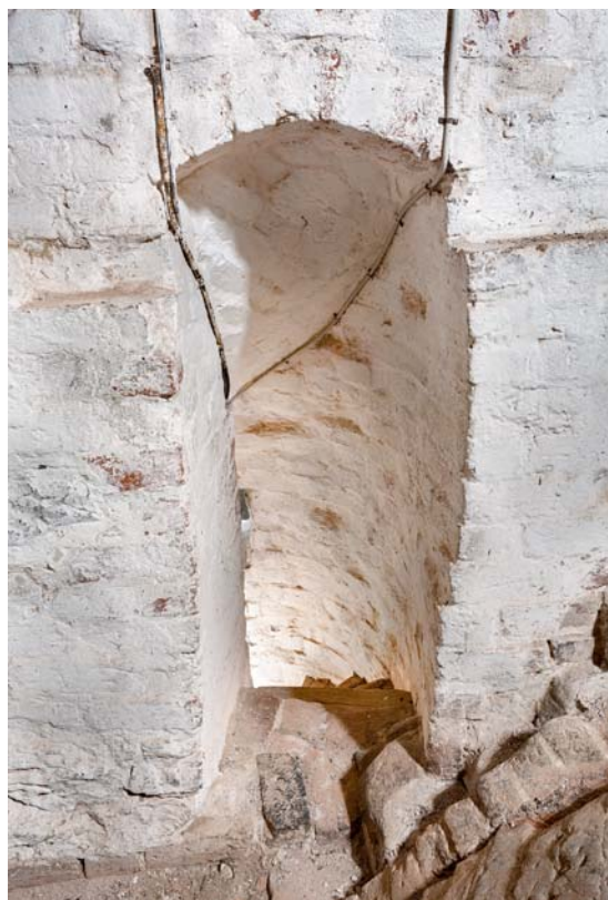
Fig. 13. Trappehusets overdør set mod syd (s. 1839). Foto Arnold Mikkelsen 2017. – Upper door of stairwell looking south.
