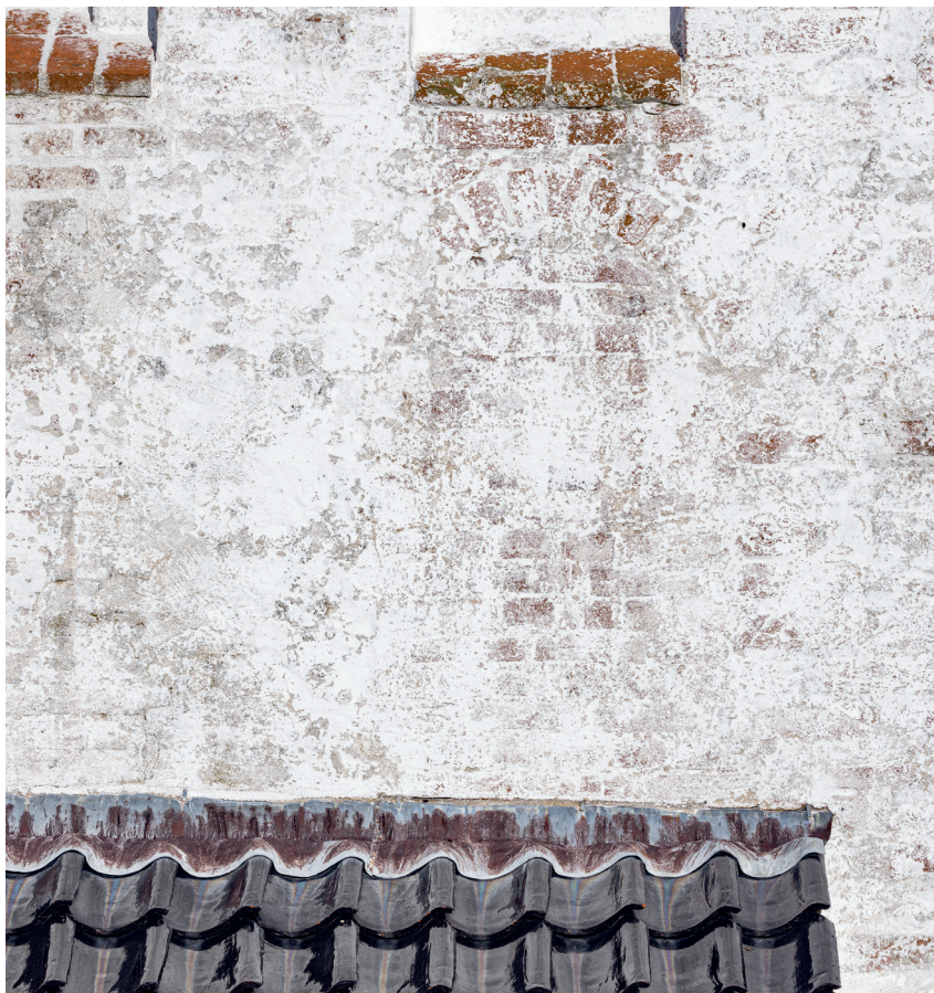
Fig. 103. Parti af tårnets sydmur med rest af murblending. Foto Arnold Mikkelsen 2021. – View of the south wall of the tower with remains of bricked-up recess.
