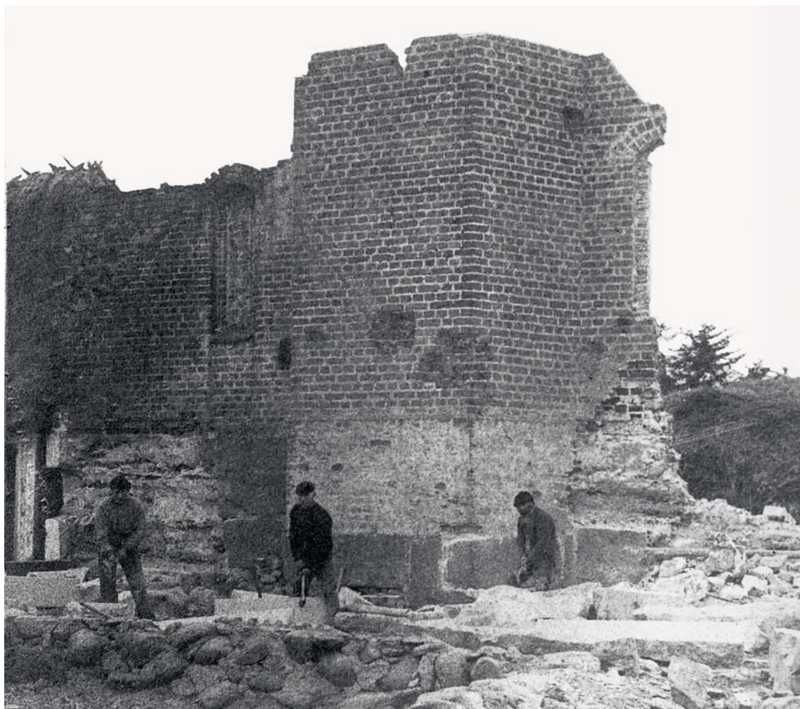
Fig. 1. Korets østmur fotograferet under nedrivningen af den tærskelade, som kirken var blevet sammenbygget med. Foto Carl Andreasen o. 1890. I Otterup Lokalhistoriske Arkiv. – The east wall of the chancel photographed during the dismantling of the barn, which the church had been joined with.
