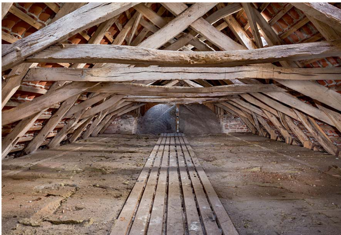
Fig. 19. Skibets tagstol set mod øst. Foto Arnold Mikkelsen 2015. – Roof truss of the church looking east.
