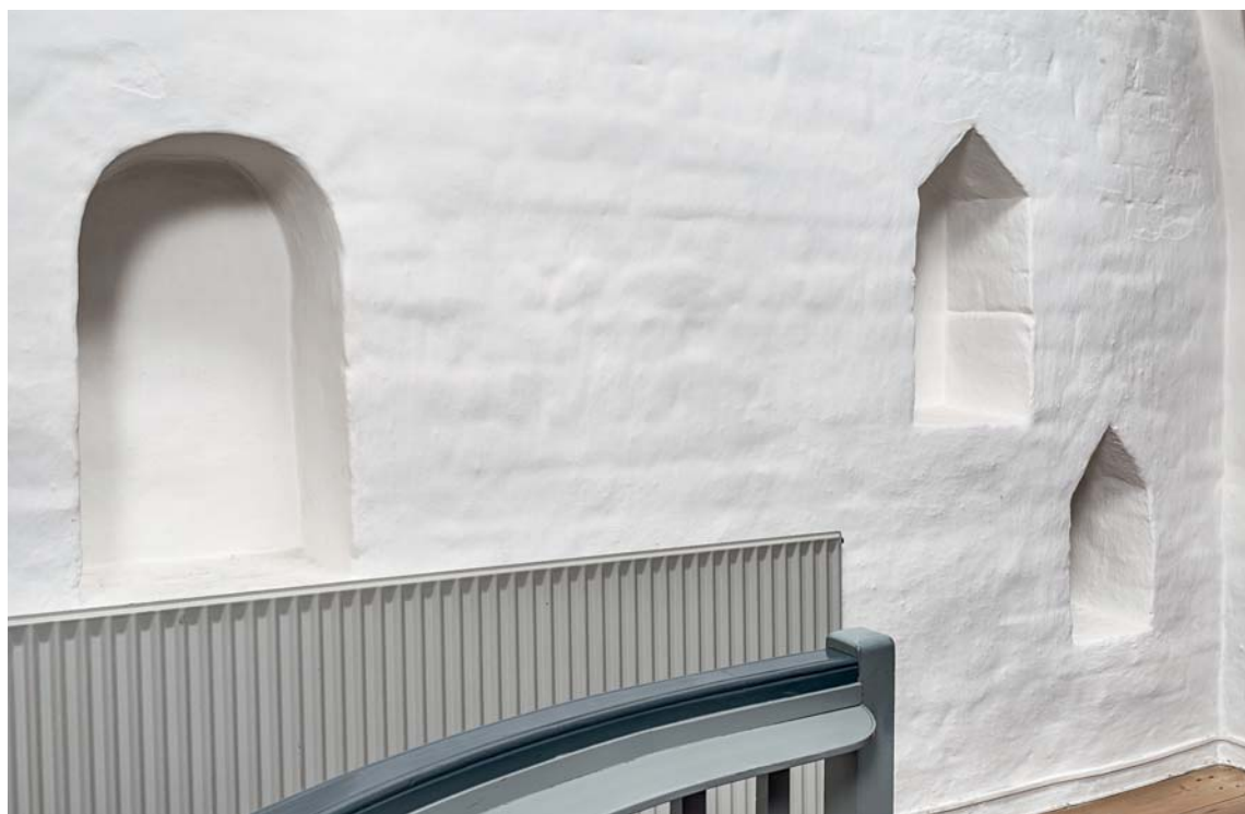
Fig. 14. Gemmenicher i korets nordøsthjørne (s. 3453, 3459). Foto Arnold Mikkelsen 2015. – Concealment niches in the north east corner of the church.
