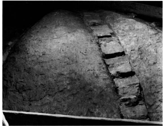
Fig. 11. Nordøstre overribbe i skibets midtfag (s. 3941). KdeFL fot. 1993. - The north-east over-rib of the vault in the second bay of the nave.
