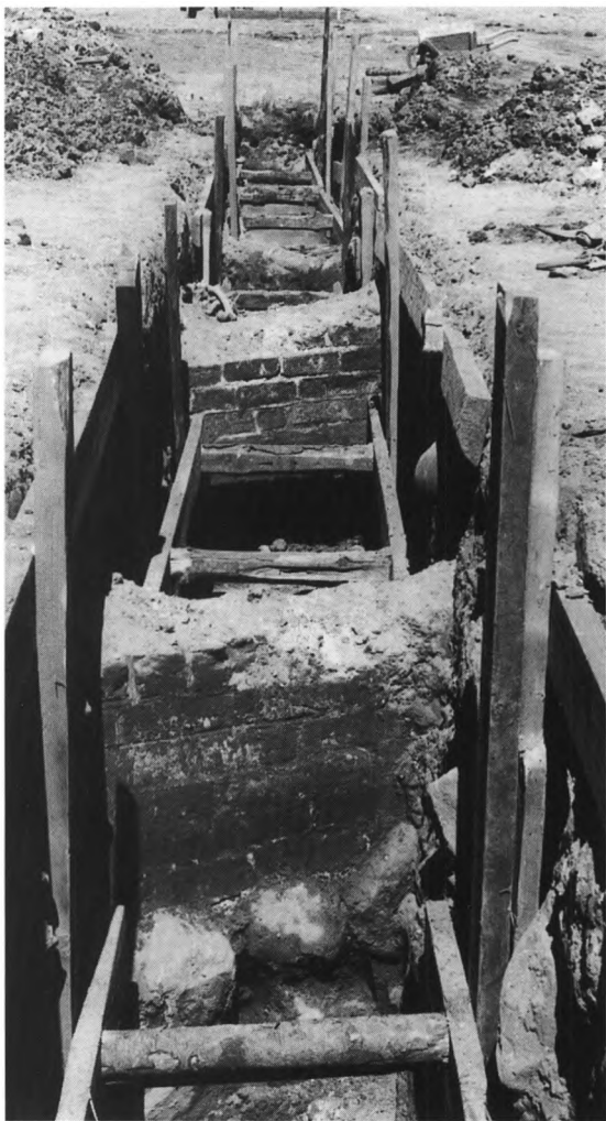
Fig. 5. Kloakudgravning i Klosterparkvej set fra syd. I forgrunden skibets nordmur (s. 3332), bagved nordmuren i søndre korsgang (s. 3332). Stadsbygmesteren i Kalundborg fot. 1948. - Drainage trench in Klosterparkvej seen from the south. In the foreground, the north wall of the nave; and behind, the north wall in the south cloister.
