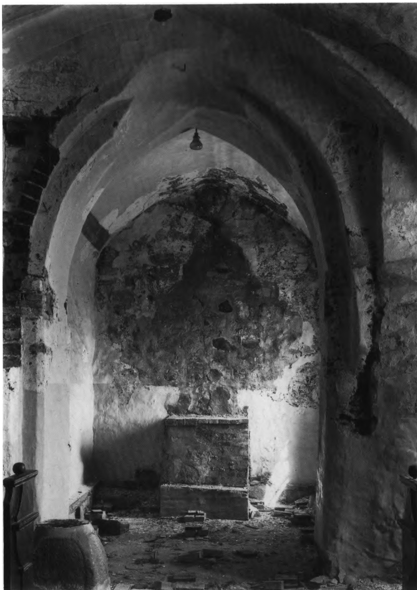
Fig. 16. Indre af \ddagger kor (s. 2529) under nedrivning. Over \ddagger alterbord ses \ddagger skyggedekoration omkring altertavle, i korbuens top udhugning til \ddagger lektorieprædikestol. Kai Uldall fot. 1925. - Interior of \ddagger chancel during demolition. Above the \ddagger alter can be seen a \ddagger shadow mural decoration round the alter-piece, and masonry hewn away at the top of the chancel arch for the \ddagger pulpit gallery.
