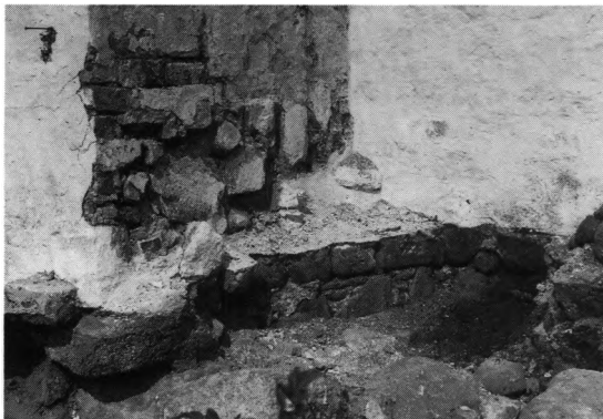
Fig. 11. Rest af rundkirkemur i søndre hjørne mellem kor og triumfmur (s. 2519). Kai Uldall fot. 1925. - Relic of round church masonry in the south corner between chancel and east wall of the nave.
