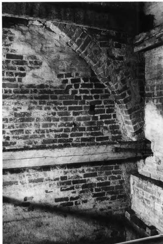
Fig. 7. Søndre halvdel af vestforlængelsens taggavl, set fra tårnets mellemstokværk (s. 1720). Over den skrå gavlkam, markeret ved aftrappet kopskifte ses udsnit af aflastningsbuen under tårnets østmur (s. 1721). Marinus Andersen fot. 0.1964. - Southern half of the gable in the west extension, seen from the tower's second storey. Above the slope of the gable, marked by a stepped heading course, can be seen part of the relieving arch beneath the east wall of the tower.
