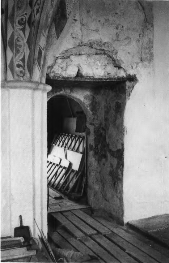
Fig. 67. Skibets norddør. Ved afbankning af pudslag under restaureringen 1966-74 sås en aflastningsbue? over den indre åbnings plankedække (s. 1766, note 21). Marinus Andersen fot. - The north door of the nave. During restoration 1966-14 when the walling was stripped of plaster a relieving arch? appeared above the planks of the inner opening.
