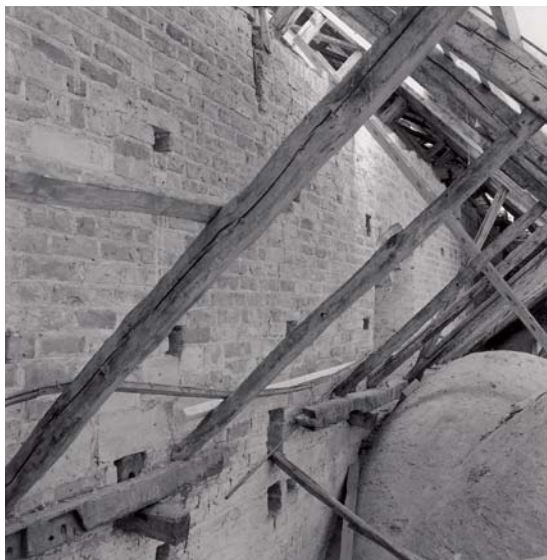
Fig. 32. Tagværk over nordre sideskib set mod vest (s. 1939). Foto HJ 1997. – View of the northern aisle's roof structure, towards the west.
